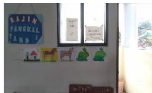
Gambar 10. Keadaan Dinding Samping
