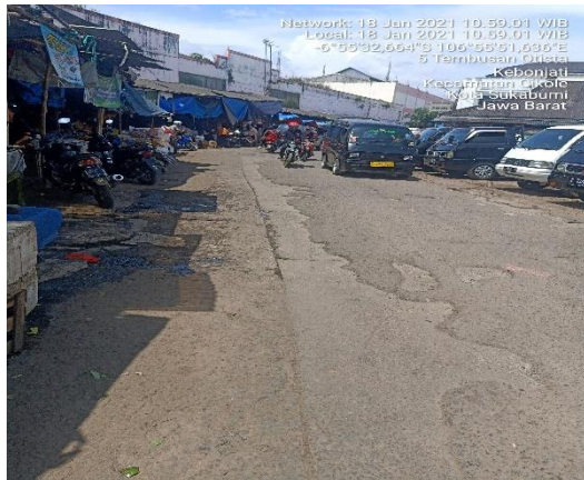
Gambar 7 Alligator Cracking (PCI) Sumber : Hasil Survei
