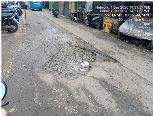
Gambar 6 Potholes (PCI) Sumber : Hasil Survey
